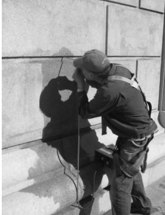
Fig. 8. Borescope examination of stone cramp corrosion.
