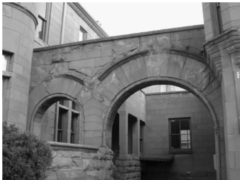
Fig. 1. Spalling, efflorescence, and surface deterioration is visible at stone surfaces between the arched openings and wall caps. Damage results from the soft nature of sandstone, water infiltration along the top of the wall, and environmental exposure. All photographs by Atkinson-Noland & Associates.
