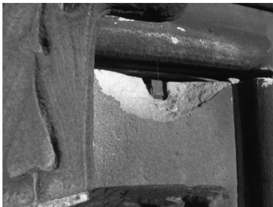
Fig. 8. Spall in sandstone unit, similar to the photograph in the ICS Illustrated Glossary showing "bursting."
