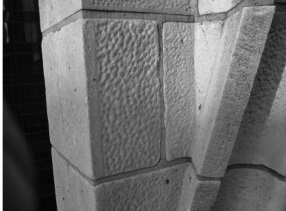
Fig. 7. Chipping at edge of marble unit, which meets the Marble Institute's definition of "spall."
