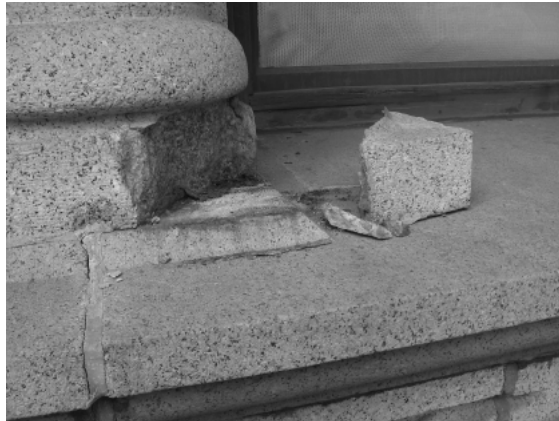
Fig. 6. Removed spall in granite.
