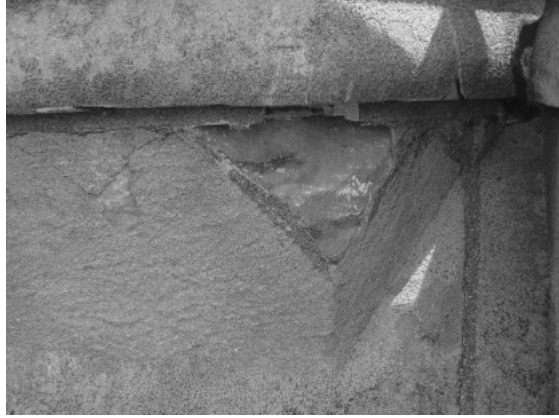
Fig. 5. Missing spall in limestone.
