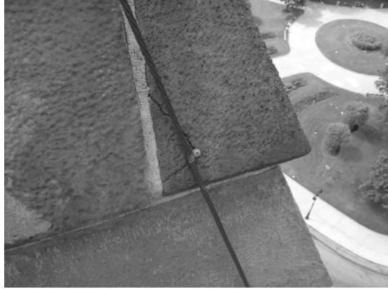
Fig. 3. Bonded spall in limestone.
