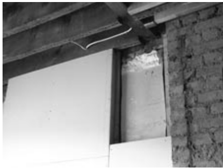
Fig. 5. Detail showing the fixing of internal insulation to the solid brick wall.
