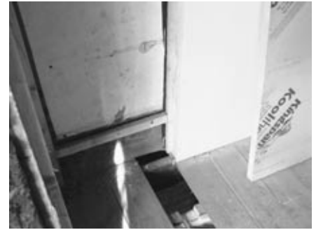
Fig. 4. The internal insulation panels are placed through the floor/ceiling interface to form a continuous, airtight barrier.
