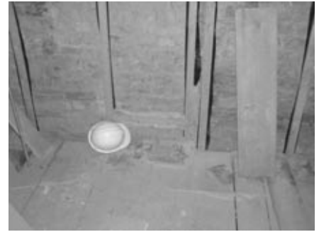
Fig. 2. At the LEVH, the demand for energy is reduced partly through a reduction in air infiltration. In this case, air infiltration is decreased through the installation of phenolic insulation panels, fixed on battens and sealed together with sealant foam.
