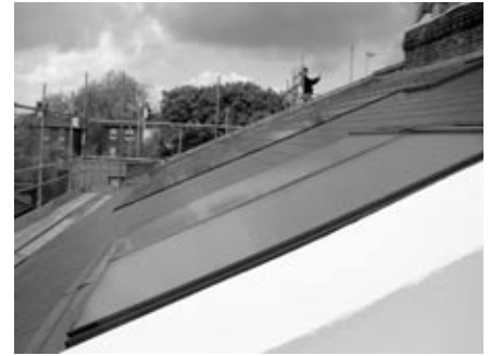
Fig. 6. The LEVH has photovoltaic panels installed on the roof for on-site generation of renewable electricity, as well as solar thermal panels for domestic hot water.
