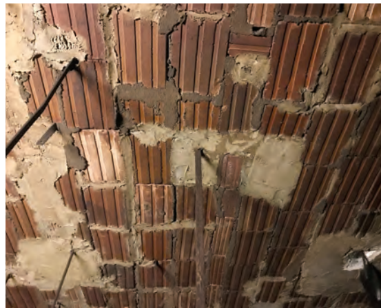
Fig. 6. Prior repairs (the light-colored mortar on the surface of the block) can be difficult to discern from “mortar slop” (dark-colored mortar) when tile arches are viewed through small probes.
