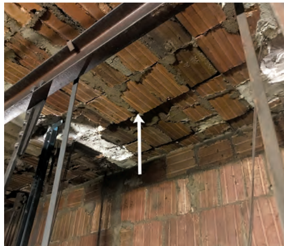
Fig. 7. Damage to the tile assembly, indicated by the white arrow, that may cause hinging in the arch may also be difficult to document where probes are limited in number.
