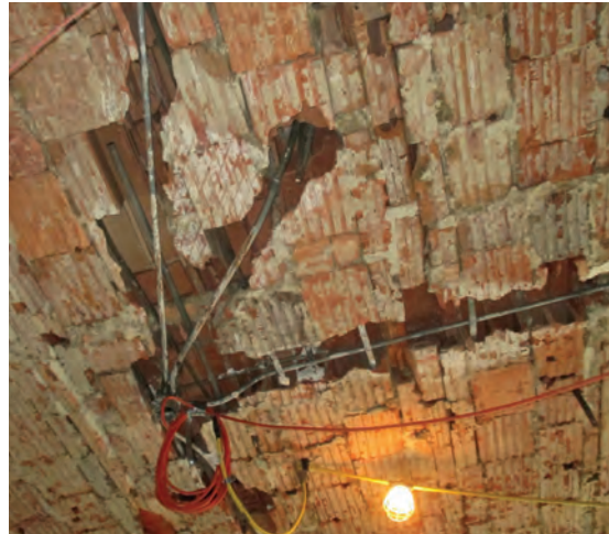
Fig. 5. Trenching through the bottom shell and webs of blocks can significantly affect the capacity of arches, as in this case, where a network of trenches was uncovered in the tiles after a plaster ceiling was removed.
