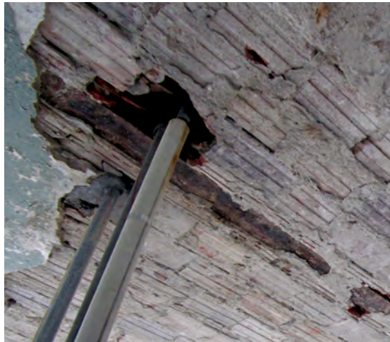
Fig. 4. Damage to tiles at a pipe penetration is frequently caused by prior chopping, rather than cutting cleanly through the arches.
