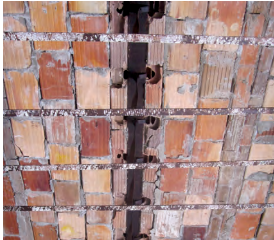
Fig. 3. Missing soffit blocks on a steel beam and pockets cut into tiles for beam clamp hangers are a common condition of systemic damage.
